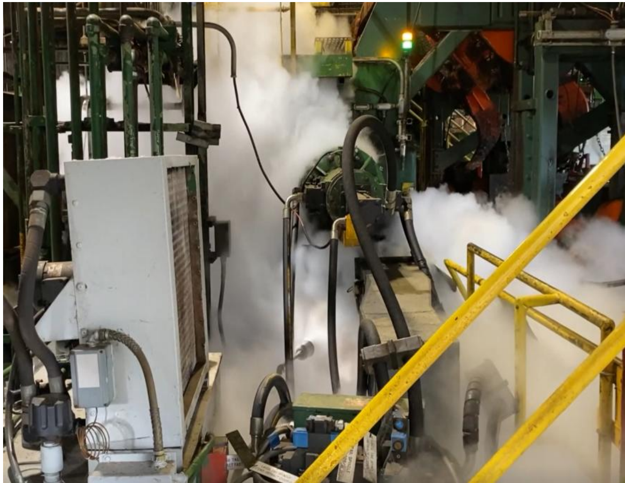
Lathe end frame view during the test discharge
