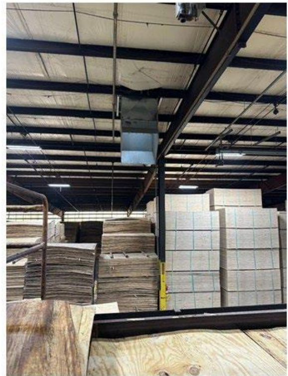
Fans ducted toward workstations
