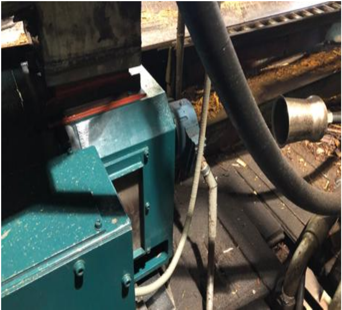
The extinguisher nozzle directed at the Lathe DC drive motor
