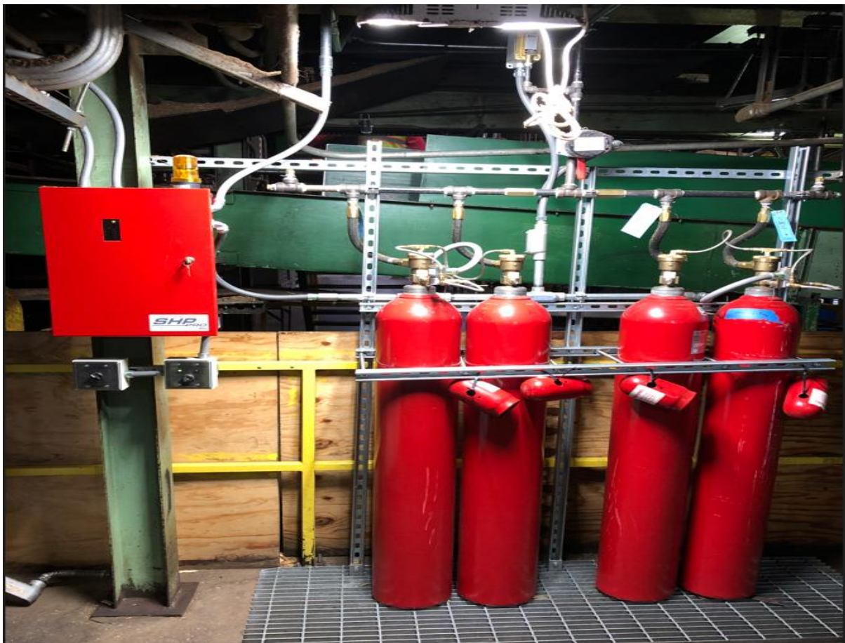
Main controller and CO 2 cylinders and back up Cylinders
